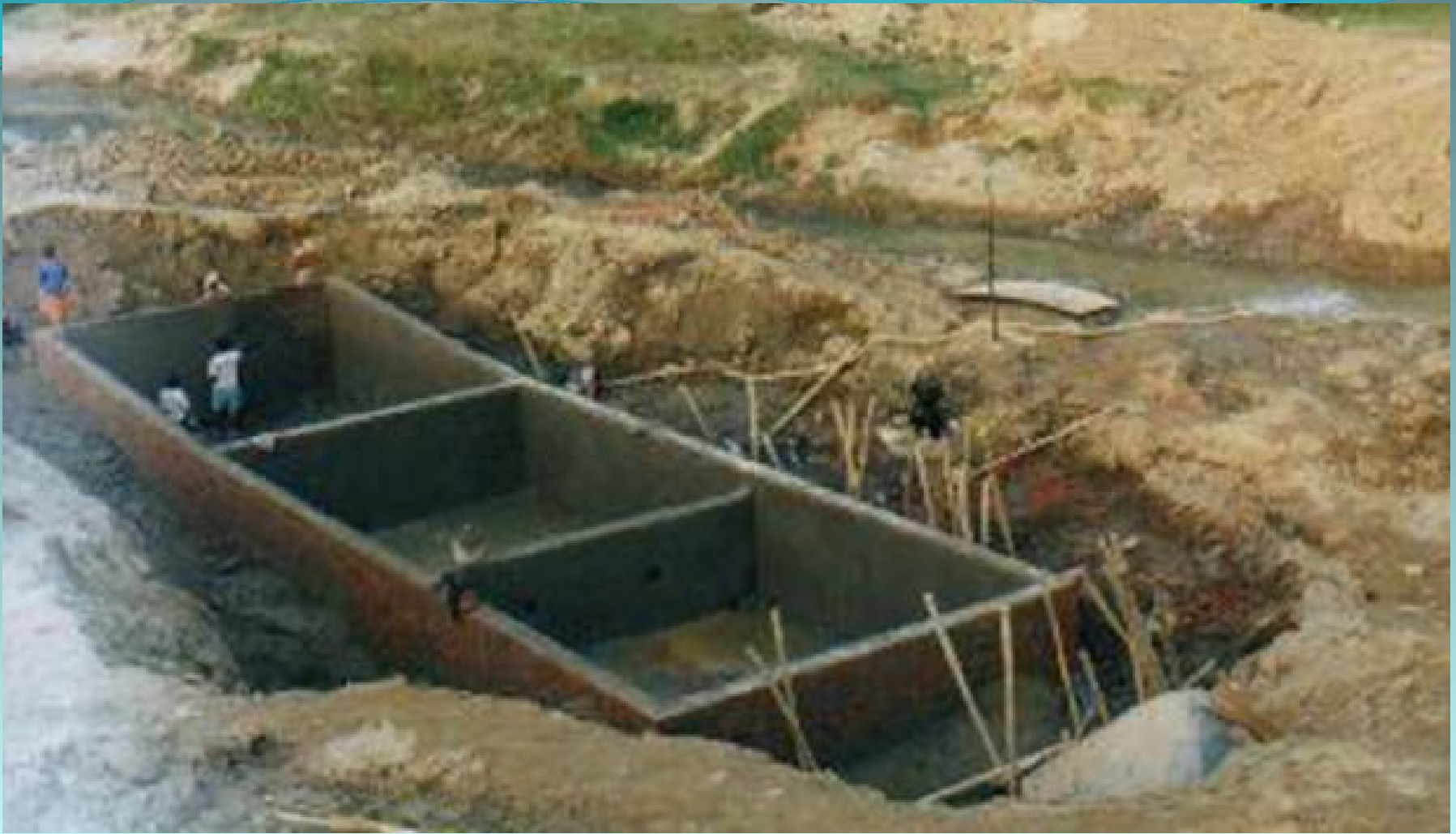
Bentonite Tank (collection+supply)
