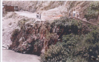
Plate 3: A close-up view of the right abutment. Note a rock cliff below the road with some overhangs and pool with eddies below the cliff. The water depth is more than 7 m. View to SW.
