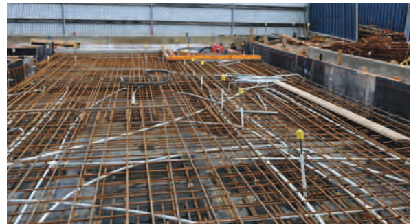
Figure 5.2 Electrical ducts cast into a slab
