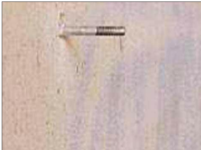
Figure 8.3: Exposed probe embedded in concrete structure
