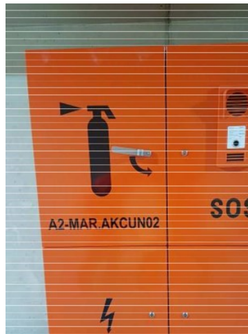
Picture 11: example of a SOS-cabinet
