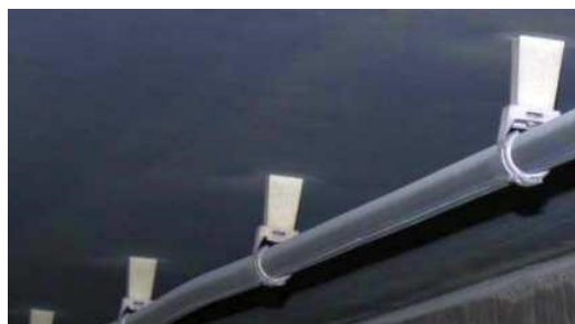
Picture 10: radiating cable
