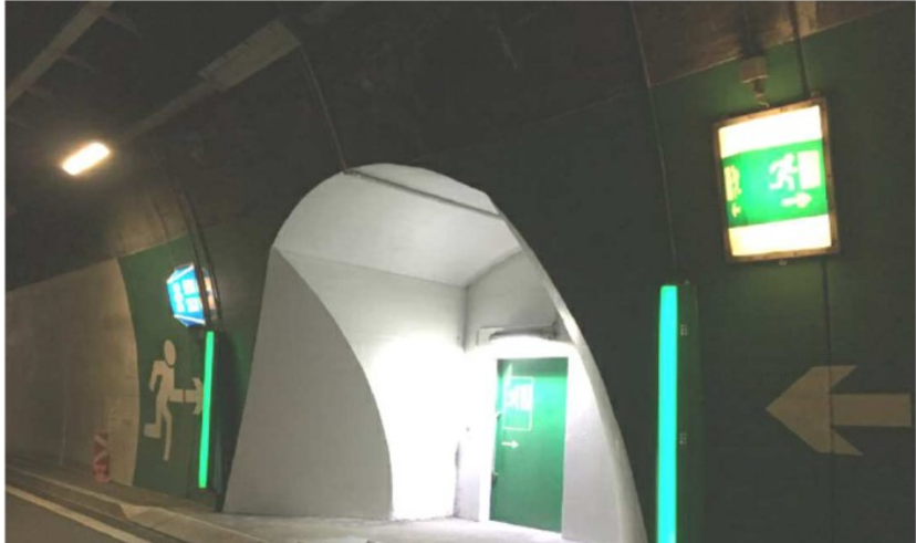
Picture 5: example of illumination of emergency exits
