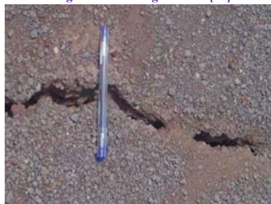
Figure D-3: Longitudinal cracking and deformation caused by expansive subgrade [11]
