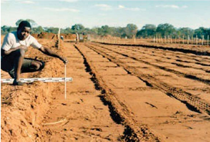
Figure D-8: Collapse settlement in excess of 150 mm following impact compaction [11]
