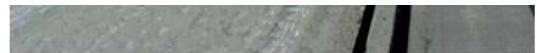
In mixed-in-place construction, cement is uniformly distributed over the area to be processed.
