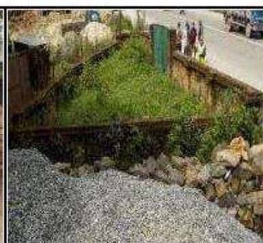
Structure No. 39: Netashwamani Dixit, Mahadevsthan 1 Kha, Plot No. 17, Brick Masonry Wall, Full Impact, 0+325, Left Side
