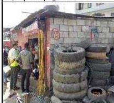
Structure No. 19: Kathmandu Oil Store and Trade Links, Mahadevsthan 2 Kha, Plot No. 2, Concrete Block with CGI Roof, Partial Impact, 0+125, Left Side
