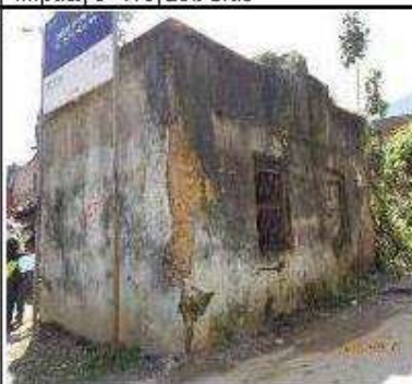
Structure No. 47: Mohan Maya Shrestha, Mahadevsthan 1 Kha, Plot No. 1, Brick Masonry and CGI Sheet Roof, Partial Impact, 0+440, Left Side
