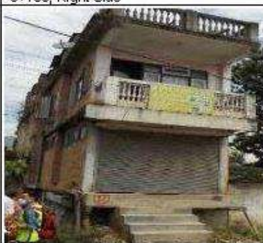
Structure No. 17: Ganesh Bahadur Nakami, Balambu 6 Kha, Plot No. 70, RCC Frame Structure, Partial Impact, 0+045, Right Side
