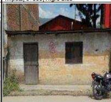
Structure No. 18: Ganesh Nakami, Balambu 6 Kha, Plot No. 70, Concrete Block with CGI Sheet Roof, Partial Impact, 0+040, Right Side
