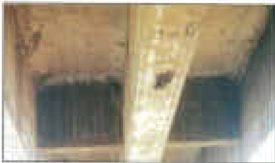
Figure 2-4: Heavy Corrosion and Spalled Reinforcement at Main Truss
