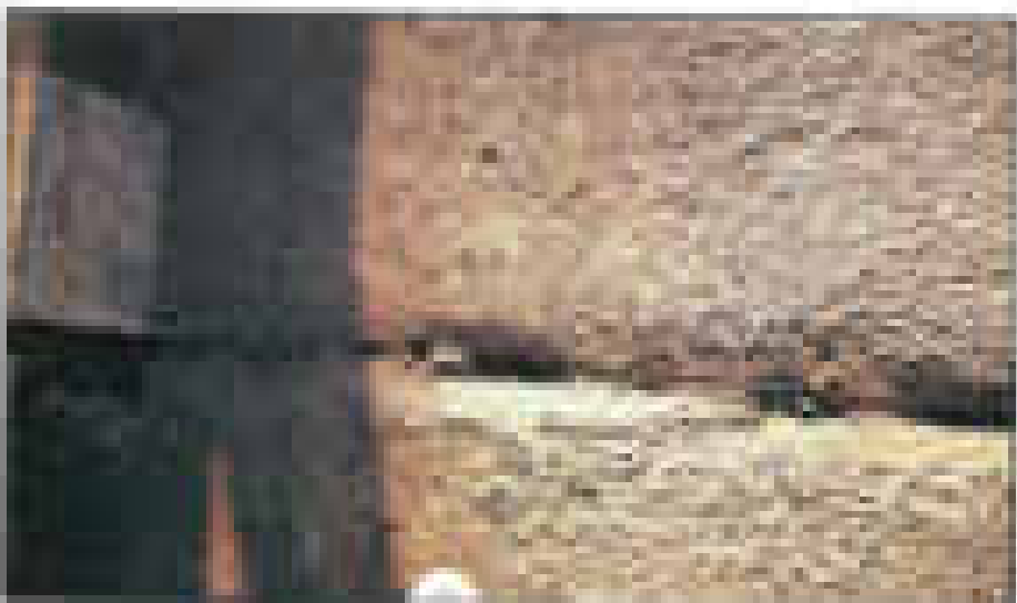
Figure 2-7: Expansion Joint needs to be replaced with roller joint movement
