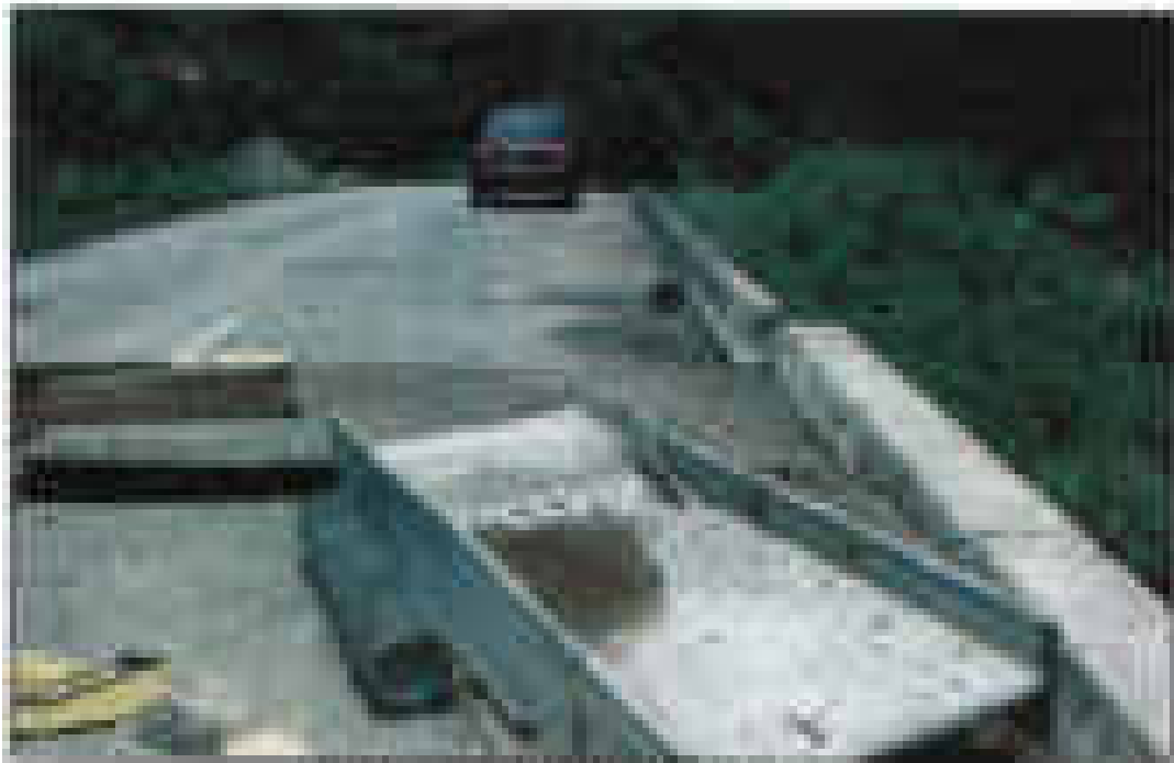
The removed damaged girder section
