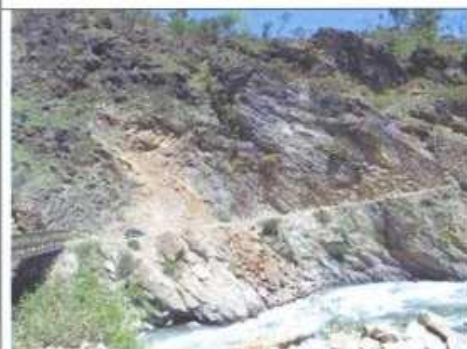
INSTABILITIES ALONG THE ROAD
