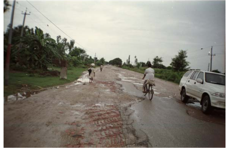
Photo 02: Road Condition at Naktajij VDC
