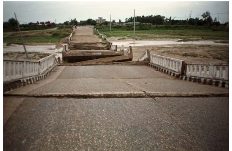
Photo 04: Collapsed Bridge at Aurahi River
