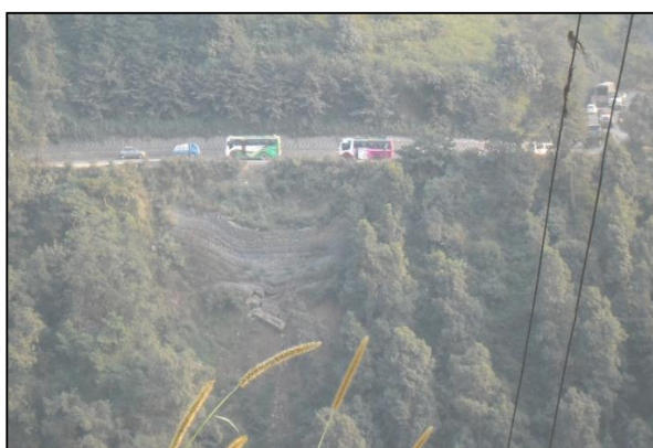
Failed gabion wall down slope of the road at Jhyaple Khola
