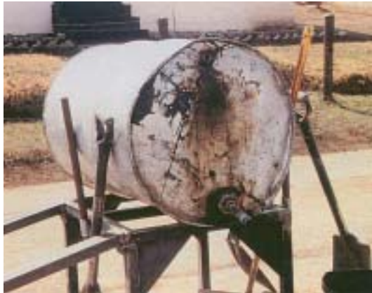
Plate 2 Stand for drum of bituminous binder.
