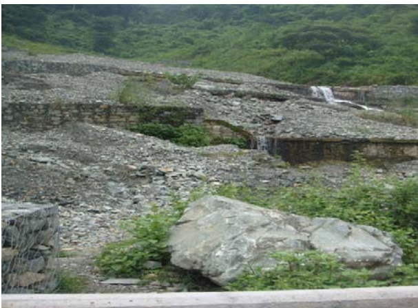
Debris deposited on check dam
