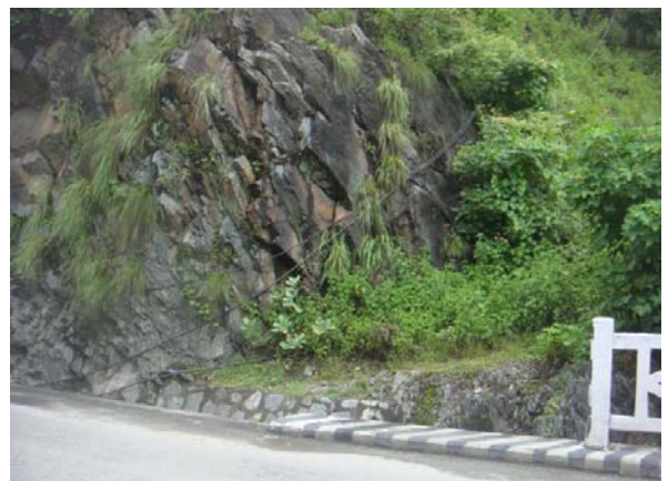
Water pipe line that could be damaged
