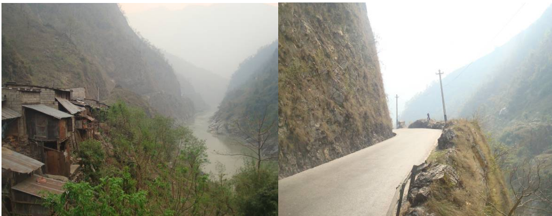
Photo 4.1 and 4.2 : Two views of the critical sections of N-M Road
