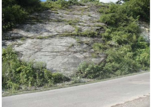
Already unstable, proper care is required
