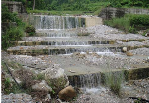
Check dam has to be improved.
