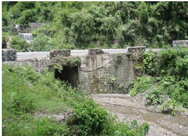
Vegetation and pipe that could be damaged
