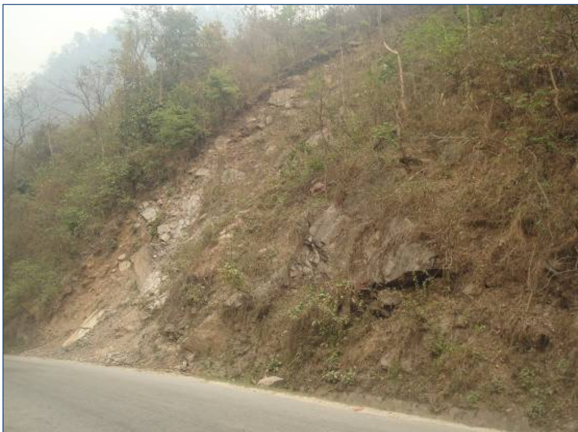
Photo 4.3 : Existing Landslide at Km 17 +800
