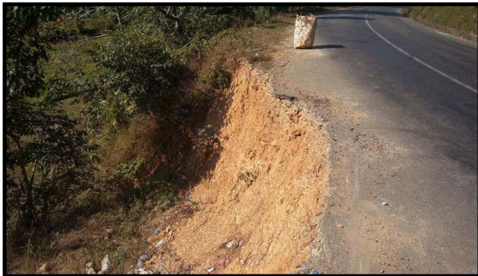
Photo 21: A minor road edge failure observed in between Ch 58+050 to Ch 58+055
