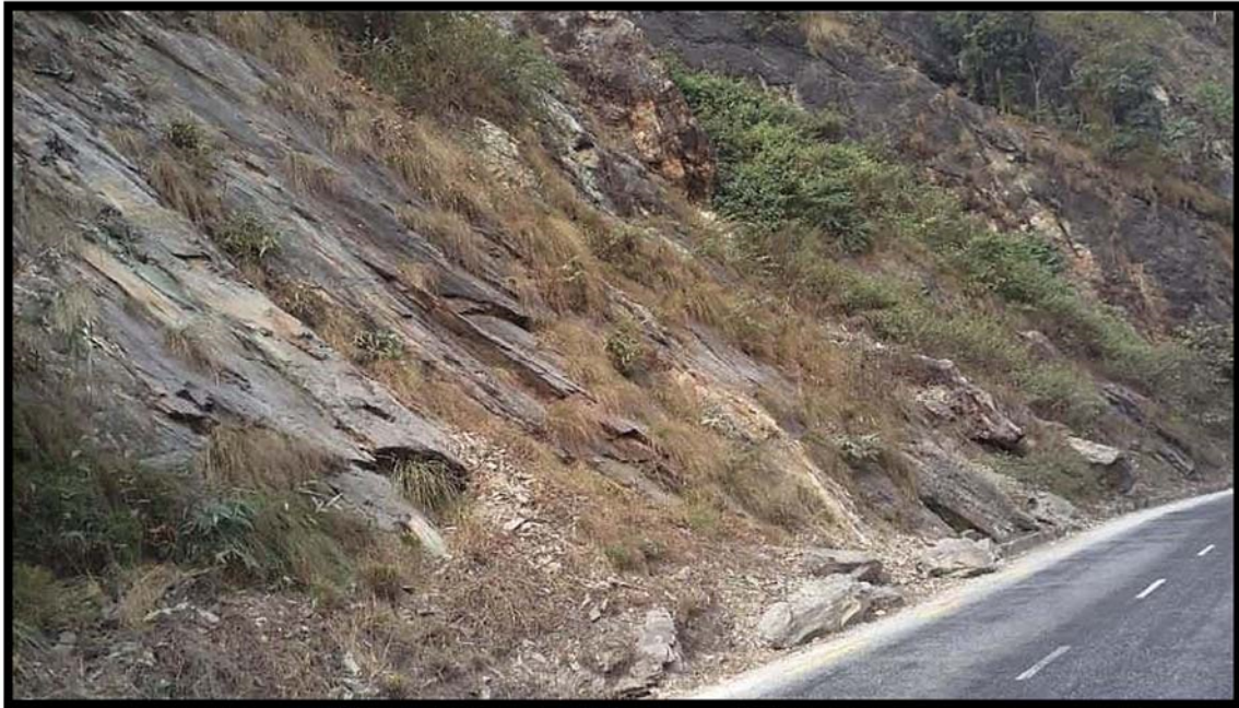
Photo 3: Rockfall observed at Ch 5+200 (planer failure)
