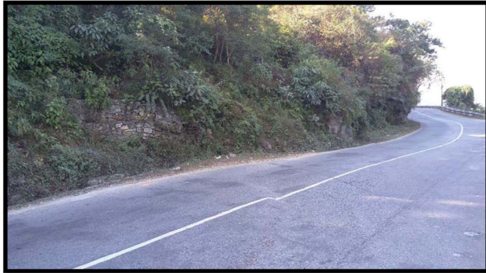
Photo 18: The subsidence of the road and gabion wall at Ch 43+050 to 43+075
