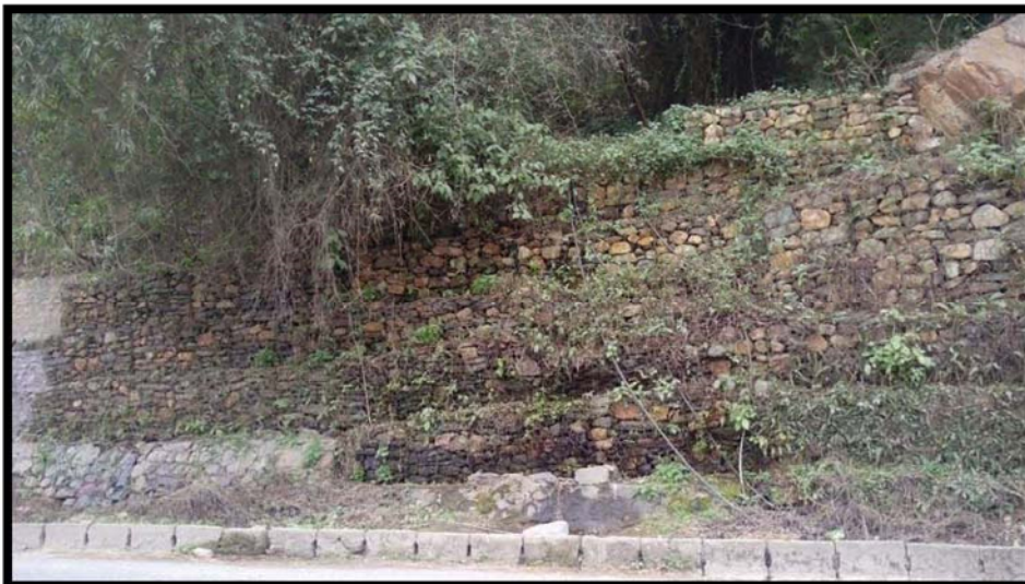
Photo 12: The bulge out gabion wall between Ch 8+850 to Ch 9+975
