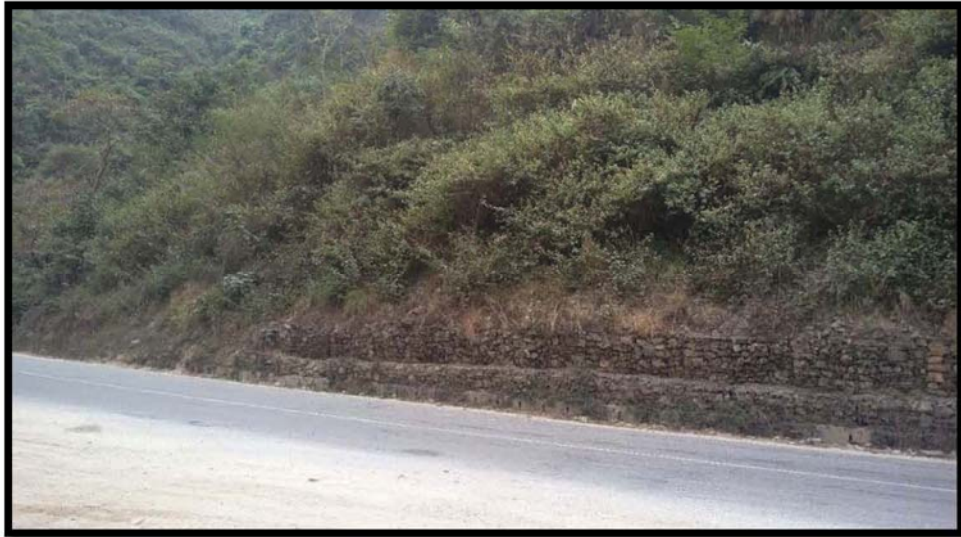
Photo 9: Bulging of the gabion wall between Ch 5+900 to Ch 6+000
