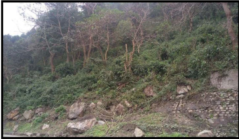
Photo 13: The slid boulder along with the retaining wall in between Ch 8+850 to Ch 9+975
