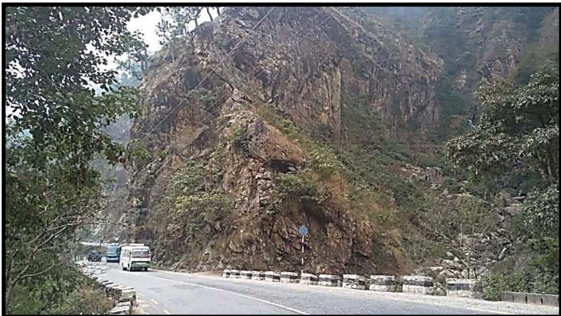
Photo 4: Jointed and fractured rockmass exposed at Ch 5+375 with possibility of wedge failure.
