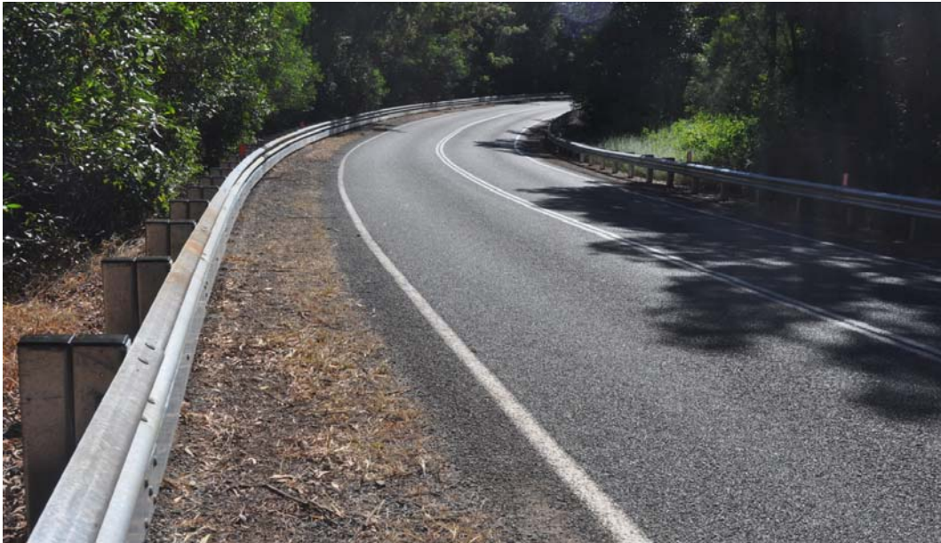
Photo 6.9: A Typical "Under Run" metal bar proposed for trial along MP Road. Also shown is the double center line marking indicating overtaking is prohibited (because it is not safe due to restricted visibility and unsafe sight distance. Also shown is the edge line (delineation measure)
