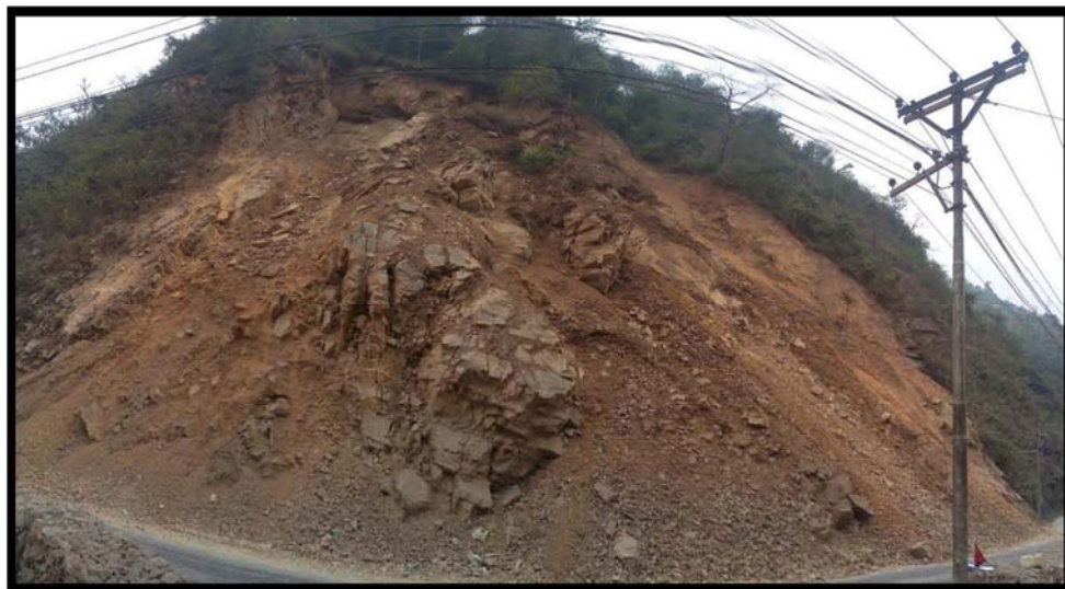
Photo 7: A major landslide between Ch5+825 to Ch 5+875
