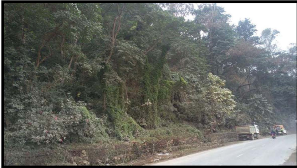
Photo 10: The colluvial cone along with the bulged gabion wall in between Ch 8+850 to Ch 9+975
