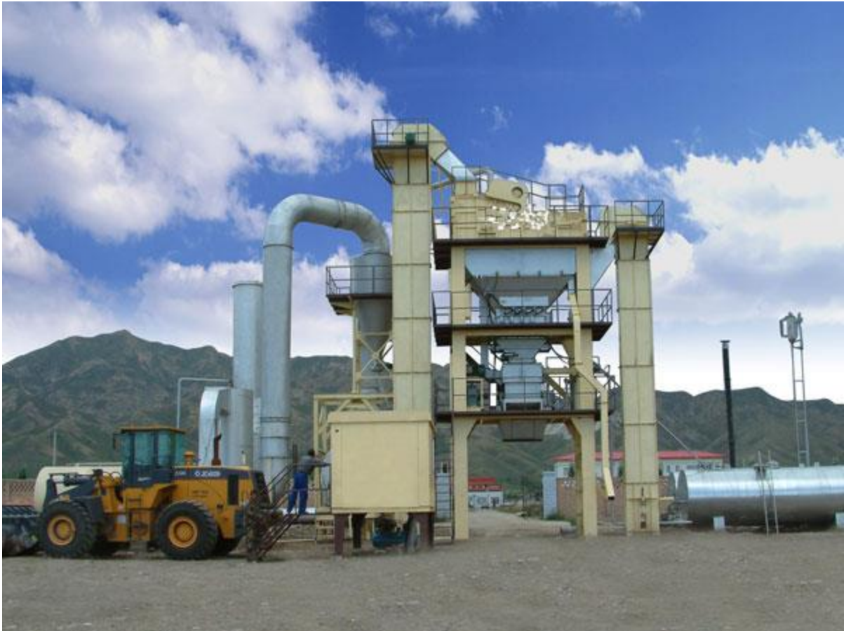
Figure 4.1 Typical Batch Plant
