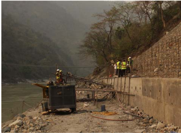
Example: Km 17 of NM road using Soil nails in river training pile structures
