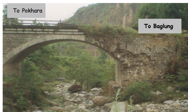
Photo 1 Damaged Armadi Bridge from upstream side
