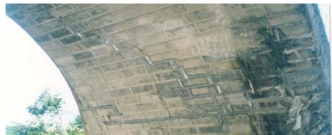
Photo 4, View of Repaired Cracks at The arch slab from below the bridge
