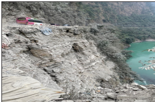
Fig. 15: Failed slope situation
