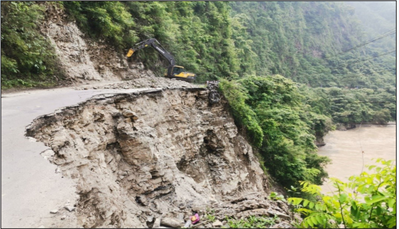
Fig. 2: Damaged Road section of Mugling-Aabukhaireni section of Road (Km 86+050), Marsyangdi River on the right-hand side
