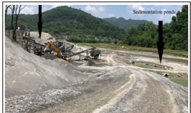
(f) Crusher plant with sedimentation ponds at MAP road
