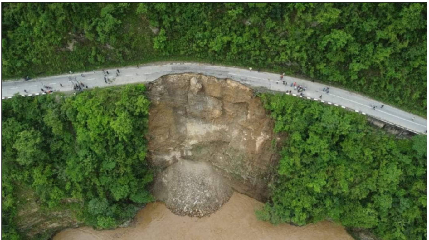
Fig. 1: Damaged Road section of Mugling-Aabukhaireni section of Road (Km 86+050)- Top View
