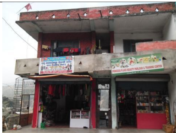
ID-49:Affected Structure of Tulasi Prasad Suyal (55+400)
