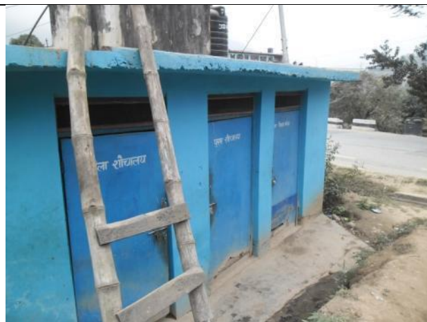
Project Affected Public Toilet at Benighat (50+950)
