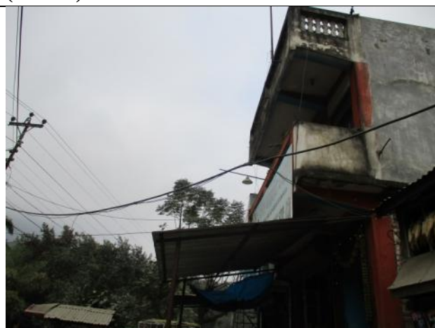
ID-76:Affected Structure of Tulsa Bhujel (73+570)
