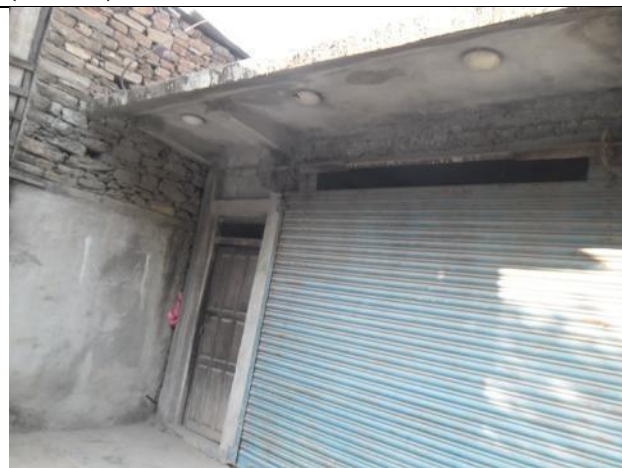
ID-20: Affected Structure of Narayan Sopkota (25+000)
