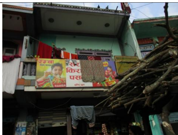
ID-67:Affected Structure of Mahendra Puri (62+050)
