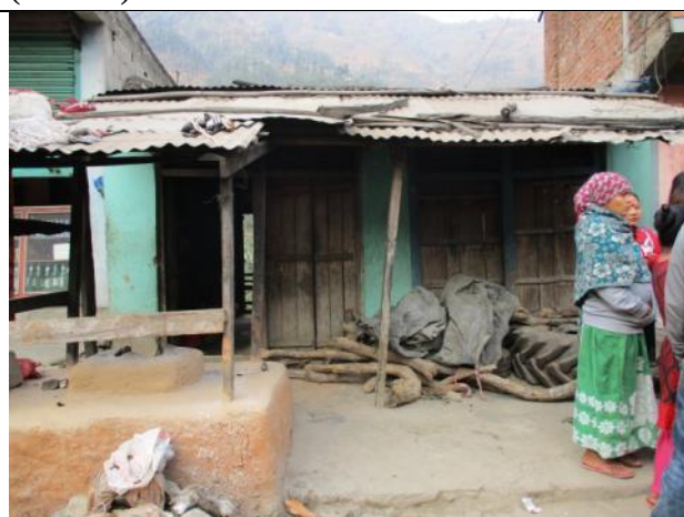
ID-69:Affected Structure of Dil Maya Chepang (62+100)
