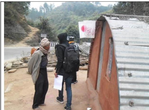
ID-38:Affected Structure of Bal Bahadur Praja (50+100)
