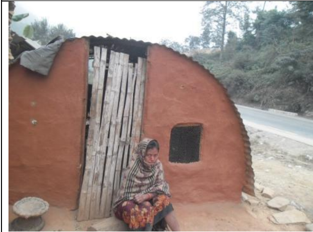
ID-36:Affected Structure of Sete Praja Chepang (50+100)
