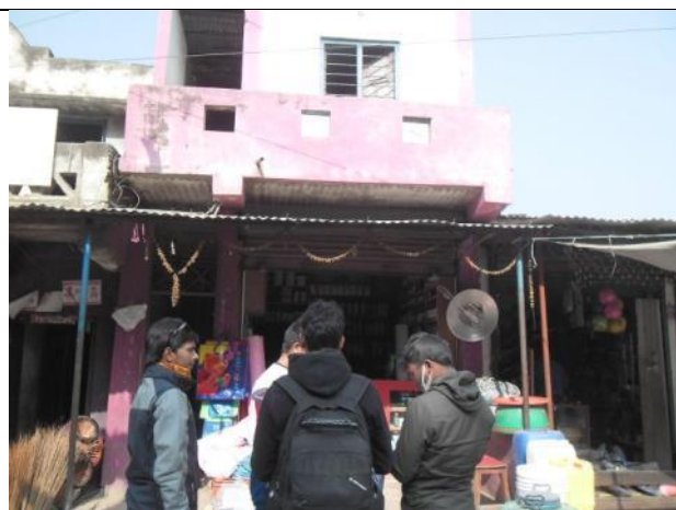
ID-55:Affected Structure of Bhim Bhadur Shrestha (55+450)
