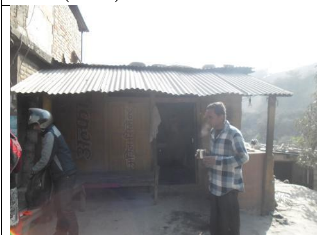
ID-29:Affected Structure of Gopal Bahadur Adhikari (26+000)
