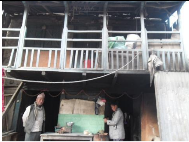
ID-21:Affected Structure of Bir Bhadur Tamang (25+000)
