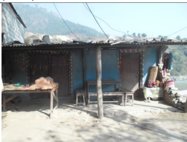
ID-32:Affected Structure of Indira Bhujel (33+000)
