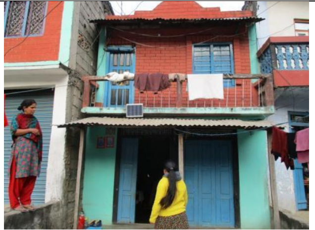
ID-65:Affected Structure of Dil Maya Ghale (62+050)
