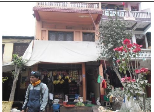
ID-42:Affected Structure of Sita Devi KC (55360)
