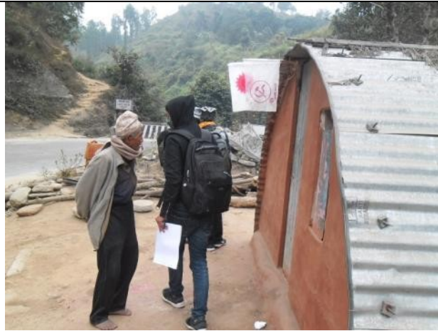
ID-38:Affected Structure of Bal Bahadur Praja (50+100)
