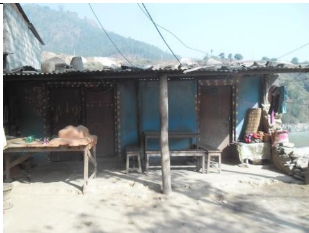
ID-32: Affected Structure of Indira Bhujel (33+000)
