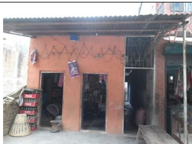
ID-28: Affected Structure of Shiva Ramtel (25+000)
