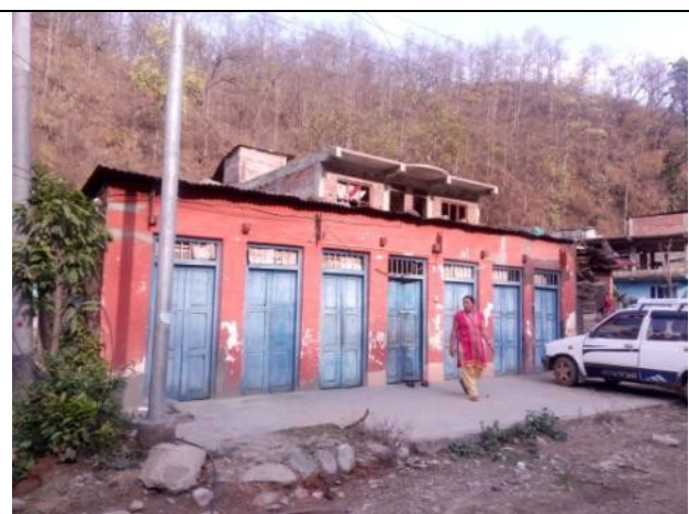
ID-18: Affected Structure of Nyarayan Dahal (23+250)
