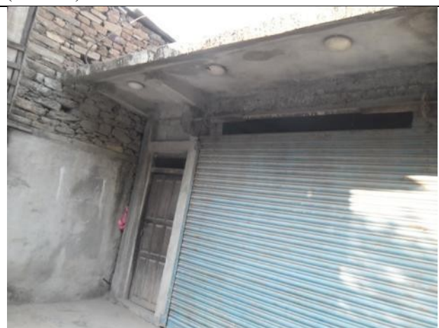
ID-20: Affected Structure of Narayan Sopkota (25+000)
