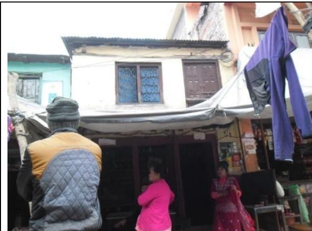
ID-43:Affected Structure of Suk Maya Magar (55+365)
