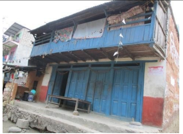
ID-73:Affected Structure of Insan Gurung (62+100)
