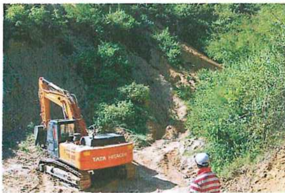
Figure 8-1: Illegal quarrying for construction industry along KNM section
