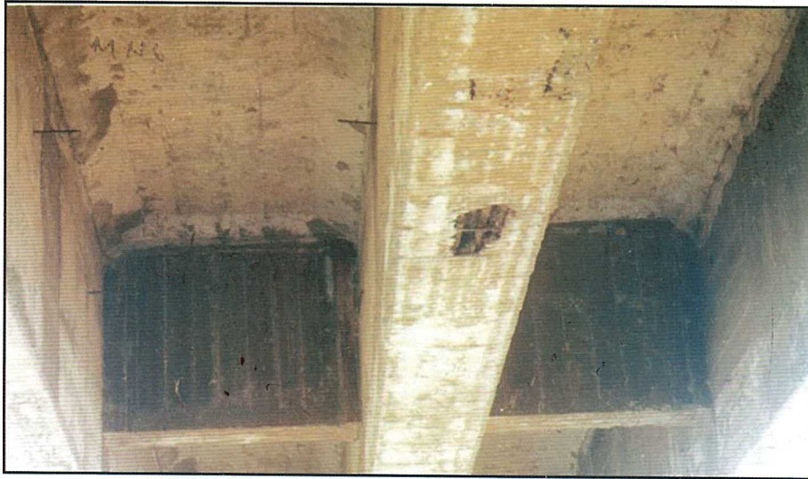
3- Honey Combs and Exposed Reinforcement on Main beams
