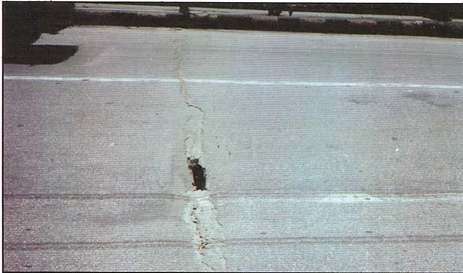
6- Missing angle plated and compression seal on Expansion joint
