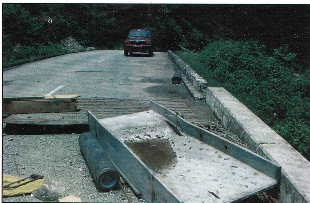
The removed damaged girder section
