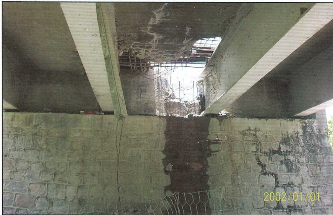
The damaged plate girders
