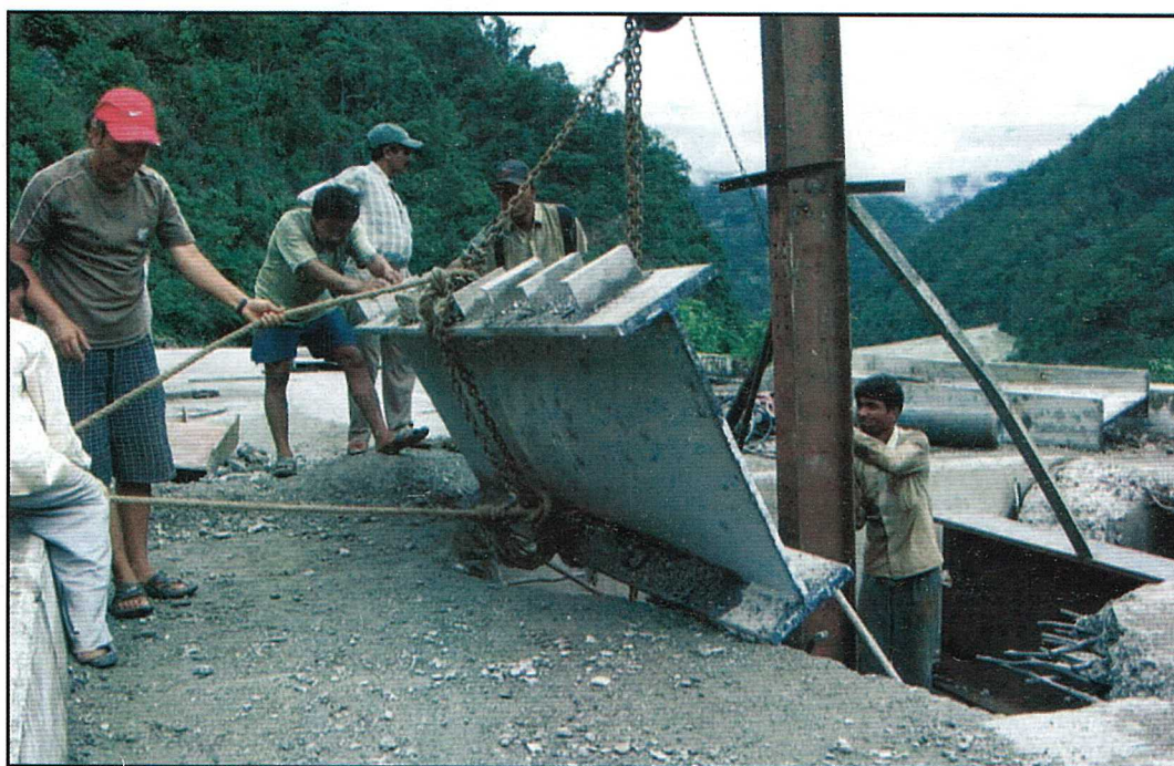
Removal of damaged girder section
