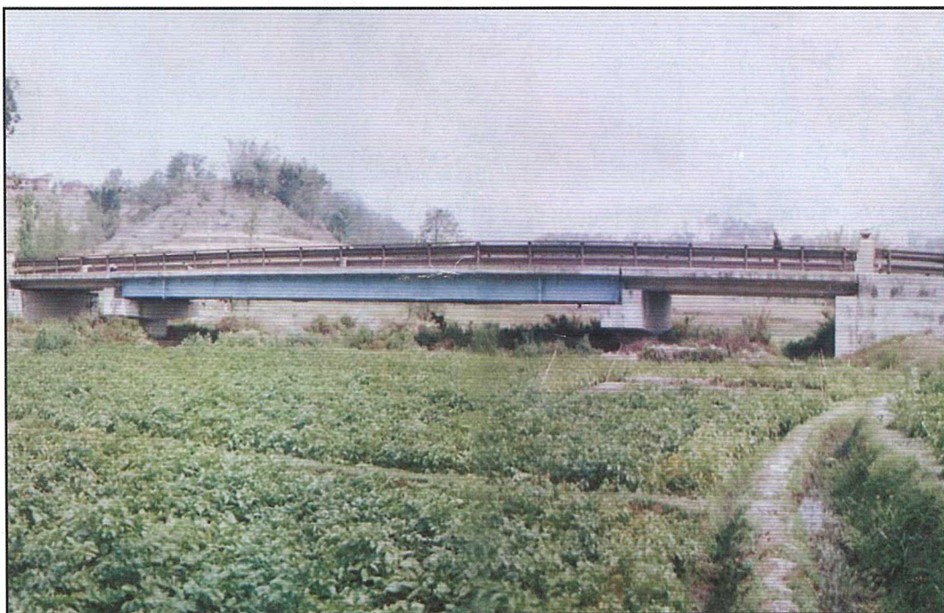
1-2 Blocked Waterway Needs clearing off
