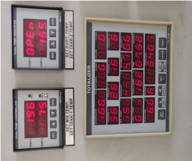
Fig. 6.10: Plant Production Control Unit Verification
