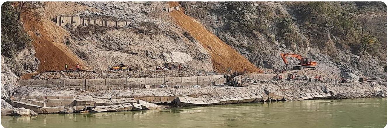
5.6 (i): State of launching apron after flood of 2021
