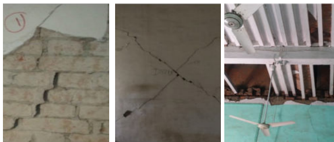
Fig. 9.3: Typical damage observed: (a) Masonry unit separation, (b) Diagonal Cracks of masonry unit, (c) Timber cracks
