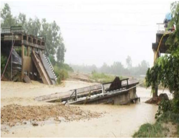
Fig. 12.2: Bridge after collapse
