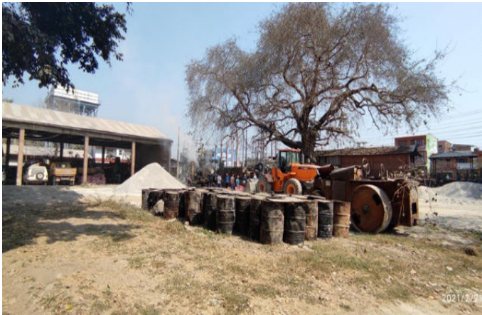
Fig. 10.2 : Material storage at plant
