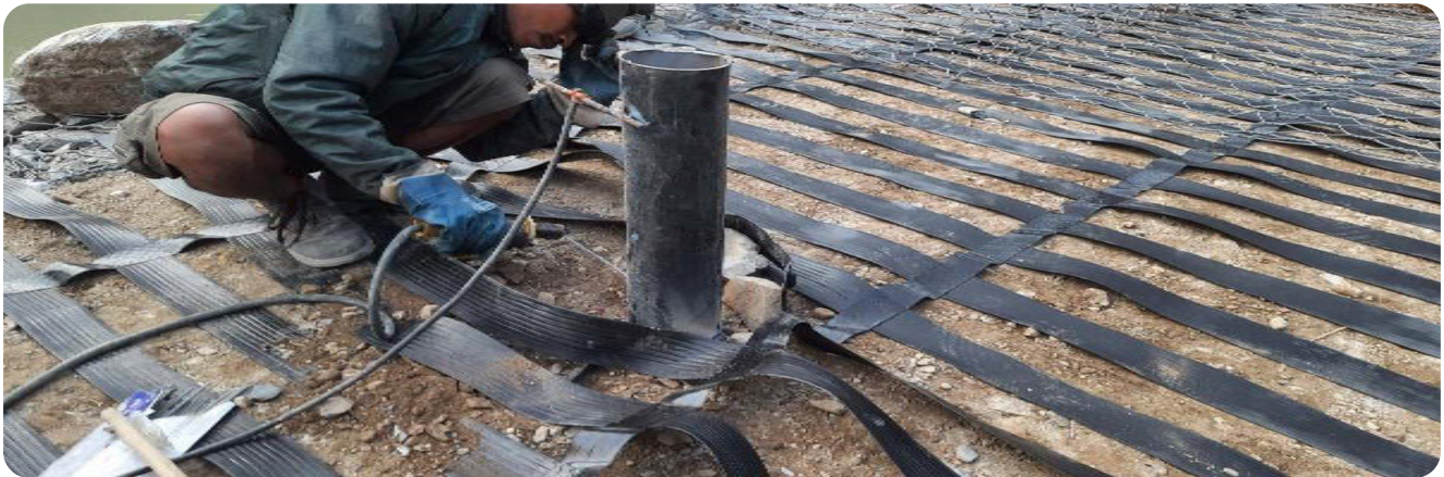
5.6 (h): Casing for piezometer
