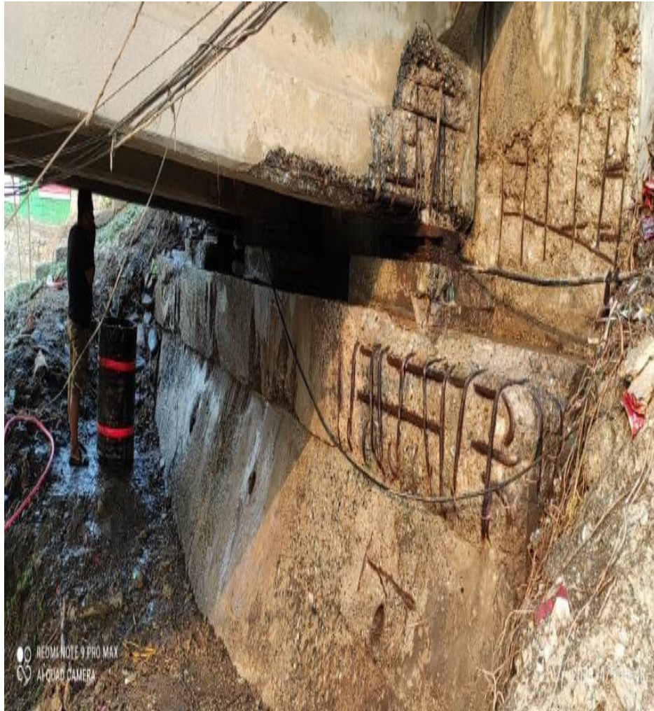
Figure 5: Exposure of reinforcement and spalling of concrete on abutment cap and dirt wall, Bakra Khola Bridge, MRM ( Before Maintenance )
