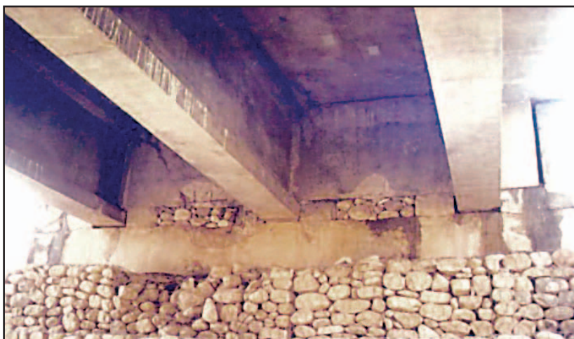
Properly maintained bearings and bearing shelves
