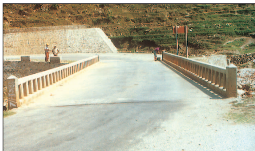
Fairly maintained Bridge signs, substructures and superstructures
