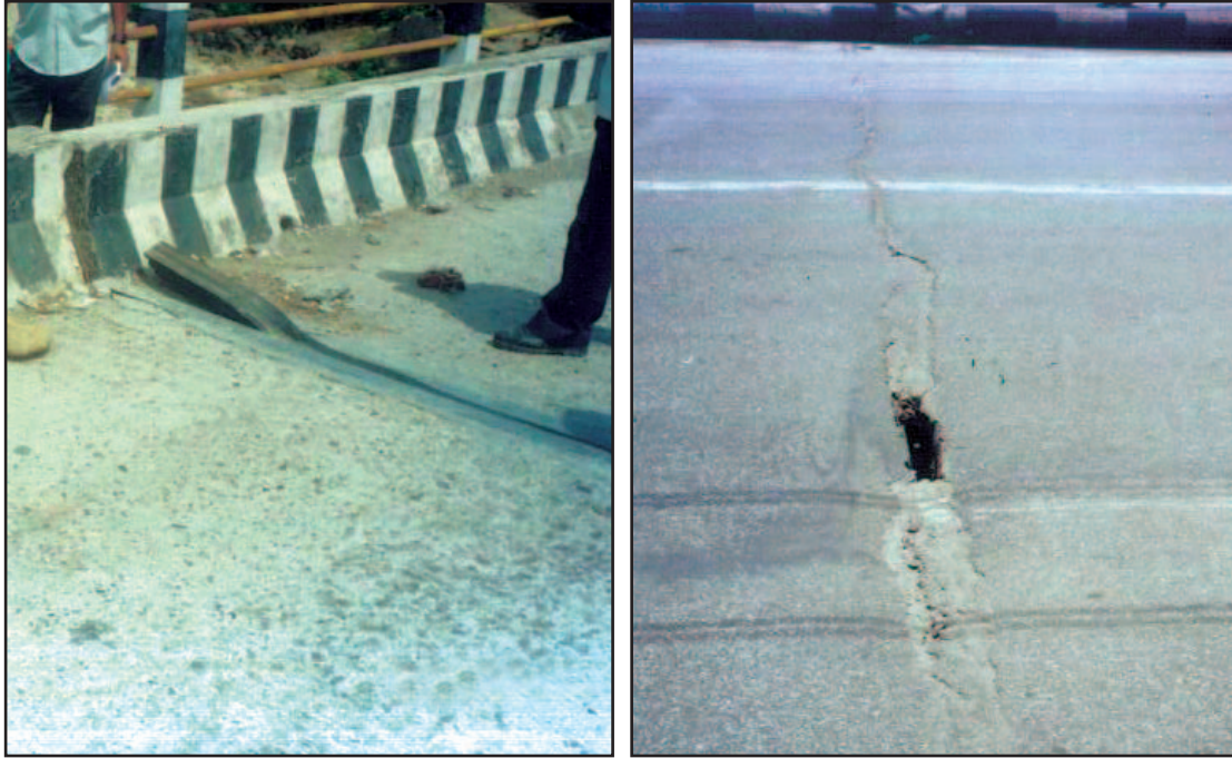
Expansion joints needed for reporting and awaiting repair
