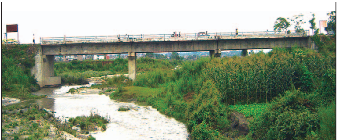
Waterway needs to be cleared, this shall be reported to Division Chief
