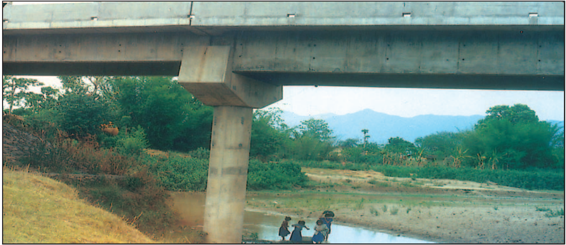
Drainage holes should be always clean as above
