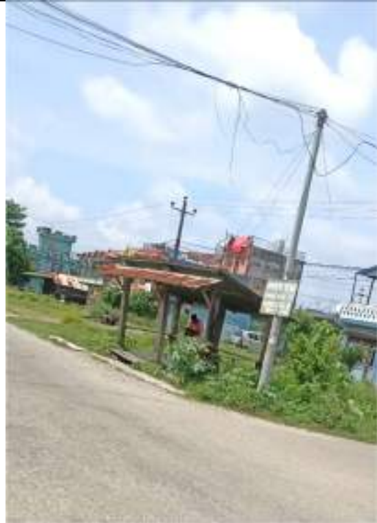
Figure 75 Poor condition of Rain shelter/Bus stop at Bangain
