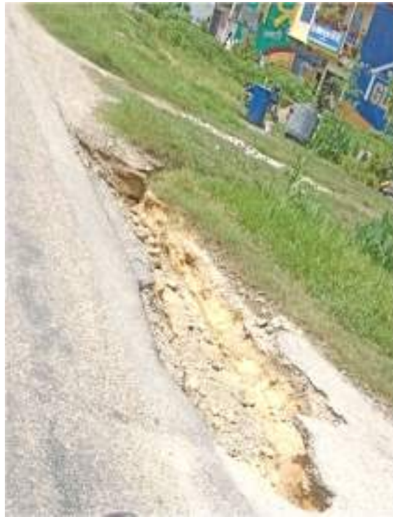
Figure 66 Unsafe Road at Murgiya
