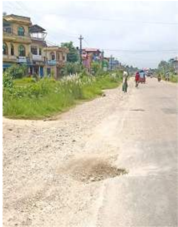
Figure 67 Potholes observed at Murgiya
