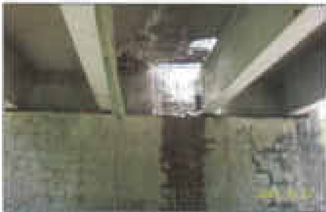
The damaged glass girder.
