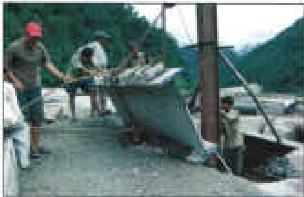
Removal of damaged girder section
