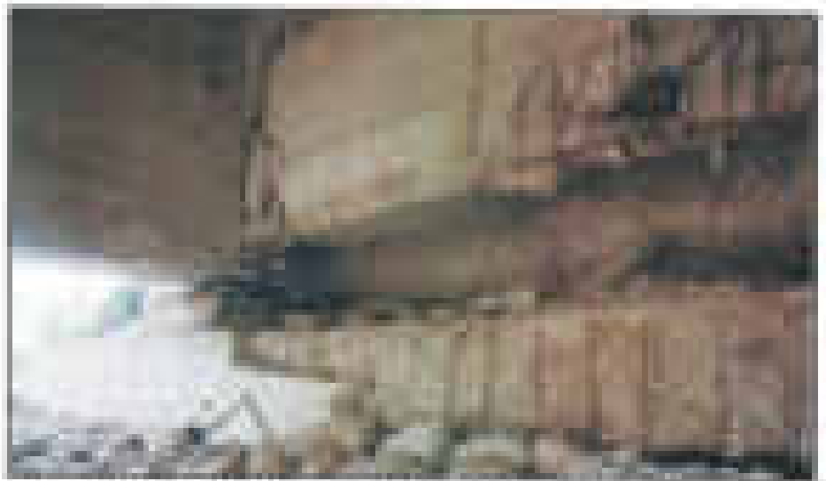
Figure 1-3: Heavy Repair Works needed at Bridge Piercap and Superstructure
