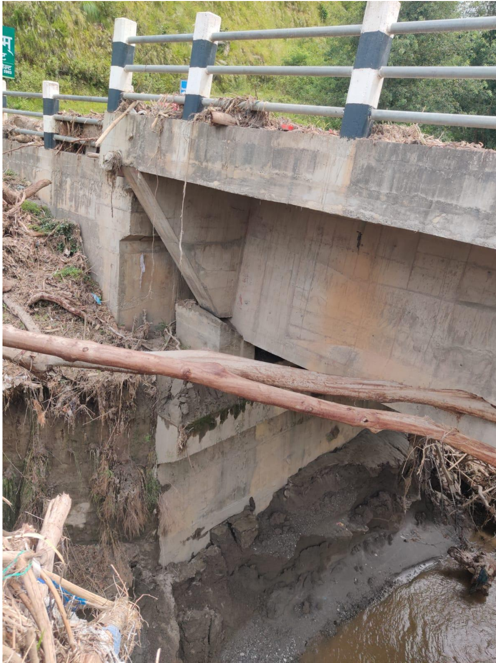
Figure 6 Shifting of Bridge deck and rest on stopper
