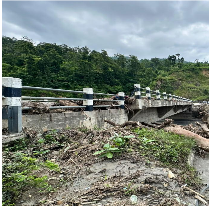
Figure 12 Overall view of the bridge and surrounding flood debris
