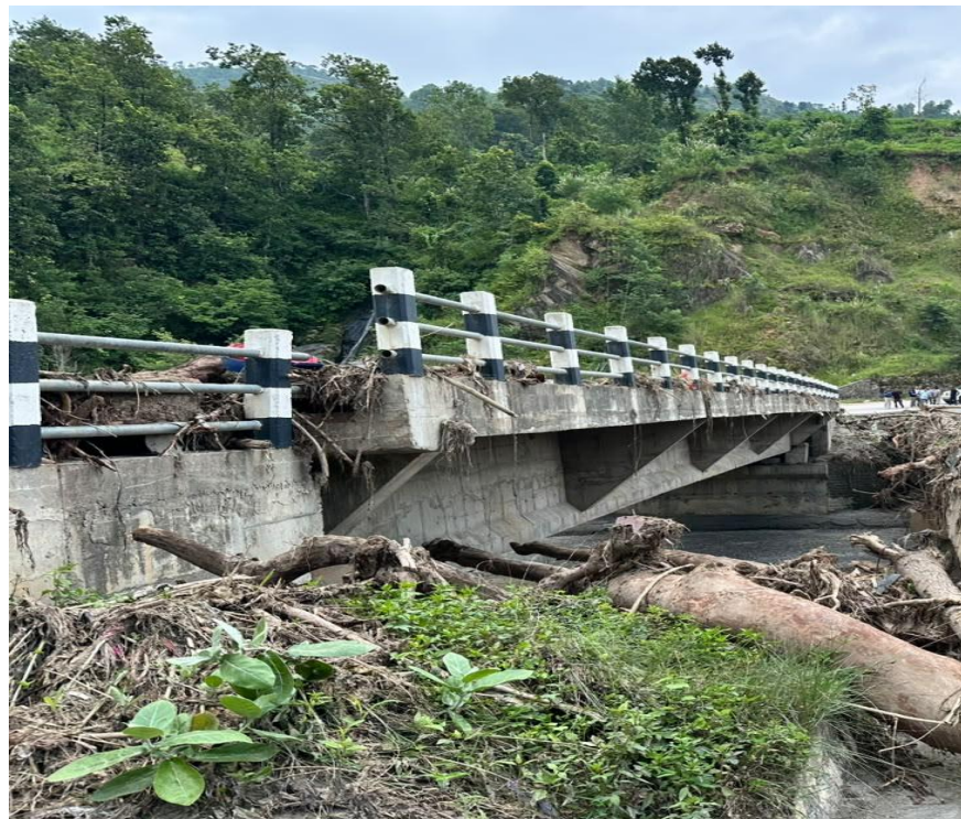
Figure 13 Bridge deck lateral shift at Downstream side
