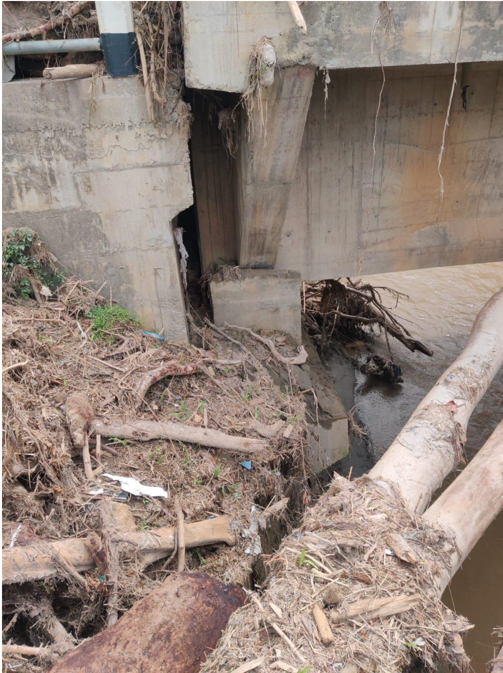
Figure 7 Close-up of abutment damage and debris near the bridge
