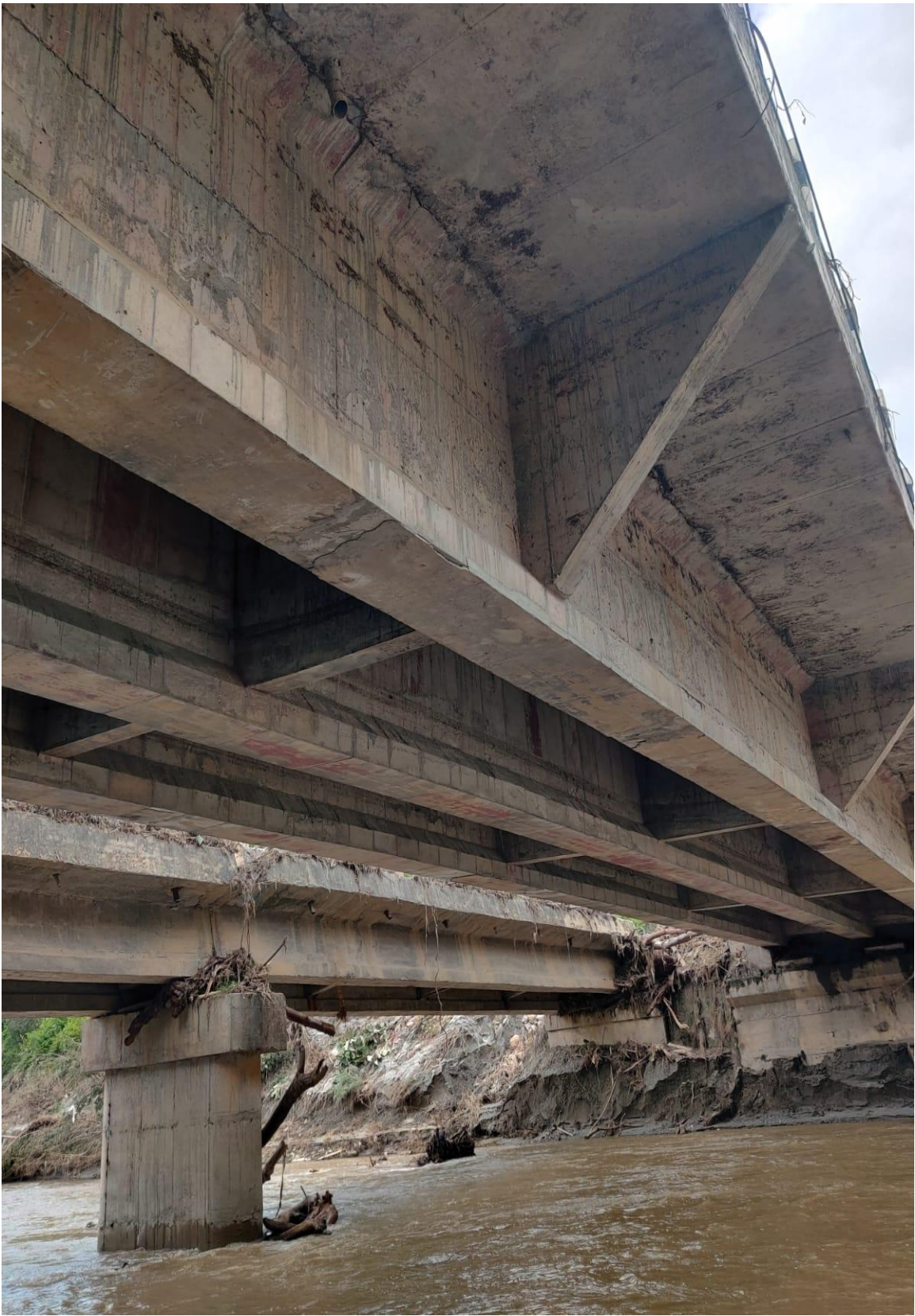
Figure 3 Underside of the bridge spanning the river with accumulated debris
